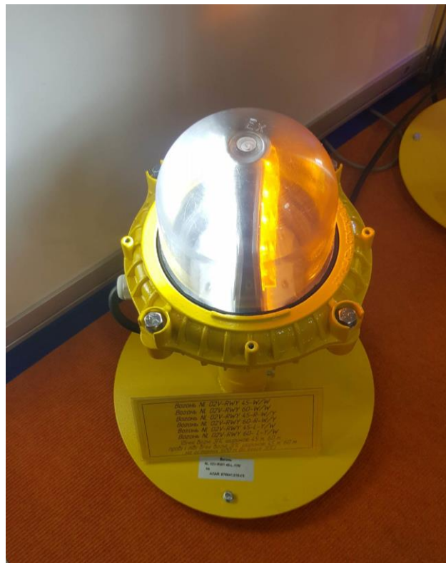
Figure 4. Ground side fire of the runway NL 02V-RWY 45-R (L) -W / Y, NL 02V-RWY 60-R (L) -W / Y
